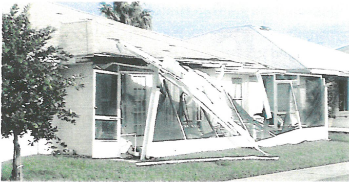
Golf course homes suffered the most structural damage from the 2004 hurricanes
